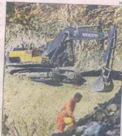
Workers making a temporary track on Monday to take machinery on top of the hill for vertical drilling in order to evacuate workers stranded inside the Silkyara tunnel in Uttarkashi for over 9 days
