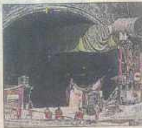
The entrance of the under construction Silkyara tunnel in the Uttarkashi district. AFP
