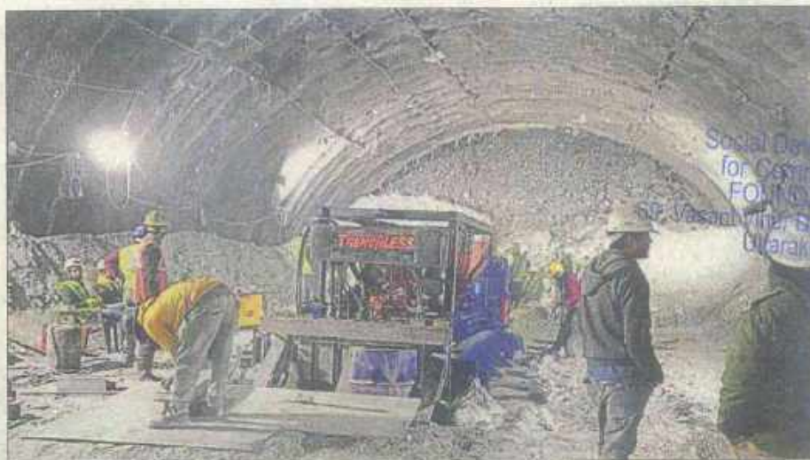
Nearly 50 metres of debris needs to be penetrated to insert the evacuation tubes.
