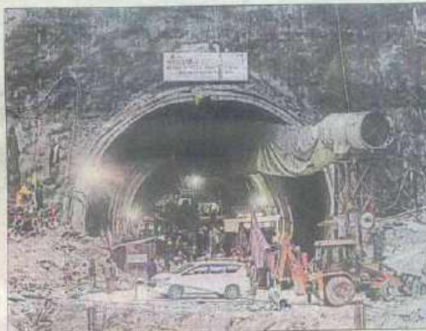
A portion of the 4.5-km-long Silkyara-Barkot tunnel caved in on November 12 trapping 41 construction workers.
