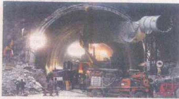
41 workers trapped in the Uttarkashi tunnel were rescued after 17 days. Chitral Khambhatil/FILE
