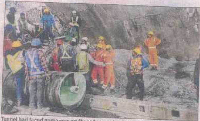
Tunnel had faced numerous cavity collapses due to the challenging geology of the region and significant rock deformation said an official
