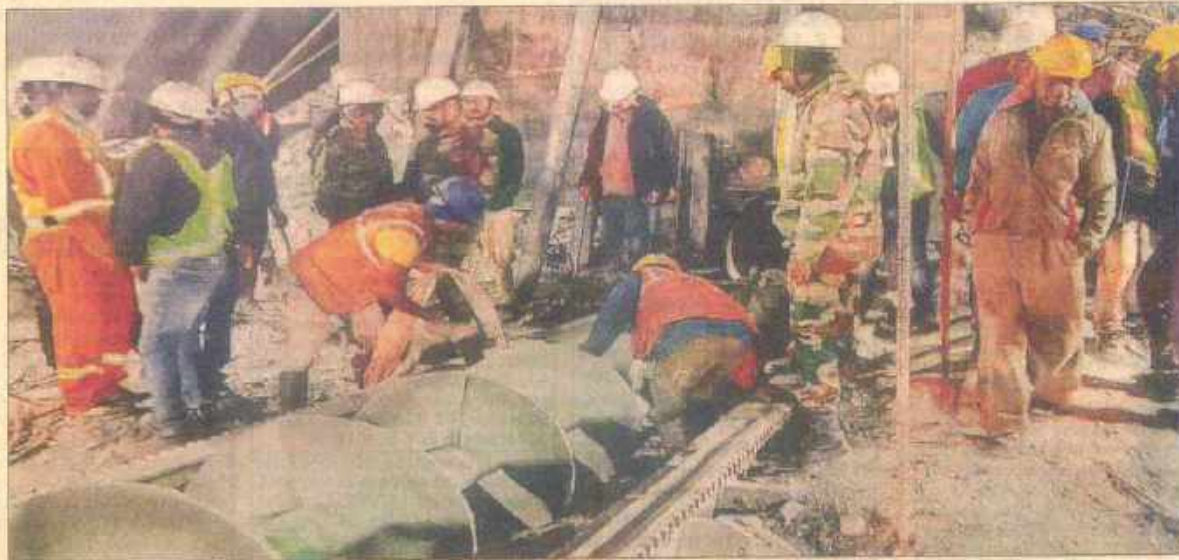
Rescue operation underway at the under-construction tunnel between Silkyara and Dandaigaon in Uttarkashi district, on Thursday
