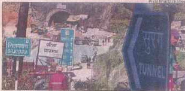
The tunnel where 40 workers are trapped for six days after a portion of it collapsed, in Uttarkashi, Uttarakhand, on Friday
