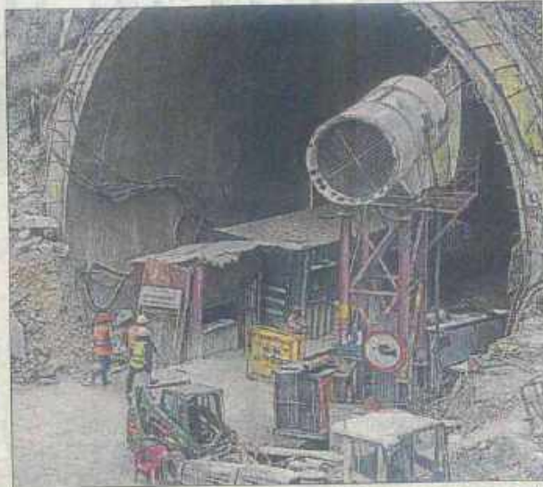
The under construction Silkyara tunnel in Uttarkashi district that collapsed on November 12, trapping 41 workers for 17 days. AFP
