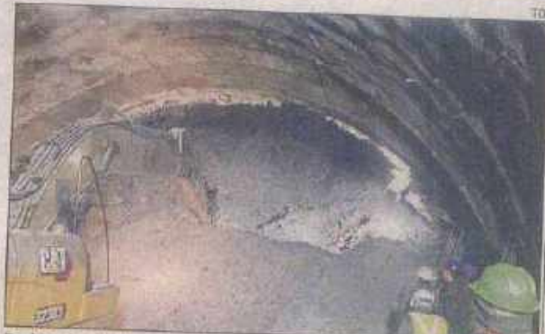
Besides food and water challenges, the 40 workers stranded inside the tunnel for past 48 hours may end up facing physical and physiological challenges, according to concerns raised by medical experts.
