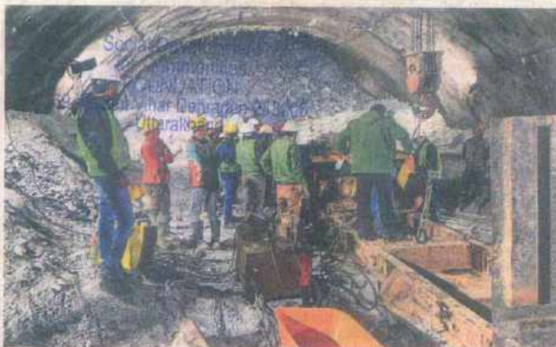
A part of the tunnel in Uttarkashi district has collapsed, walling up the passage. PTI
