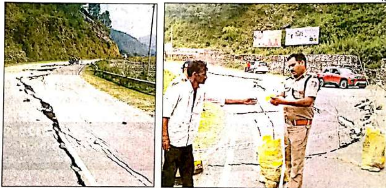
A 70m stretch of Badrinath highway between Maithana and Pursari in Chamoli district developed major cracks on Thursday, after which the area was sealed as a precautionary measure
