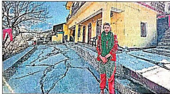
The authorities are waiting for the report to decide if starting the work again would aggravate the land crisis problem. P71
