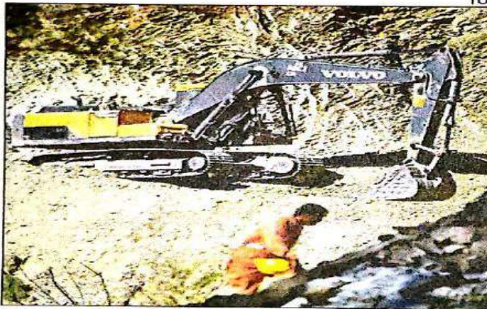
Workers making a temporary track on Monday to take machinery on top of the hill for vertical drilling in order to evacuate workers stranded inside the Silkyara tunnel in Uttarkashi for over 9 days
