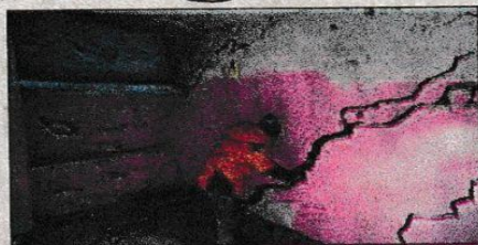
In 2023, large cracks appeared in houses in Jyotirmath. AP
